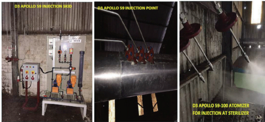
Figure 2. D3 Solution's skid and injection points at the steriliser.
