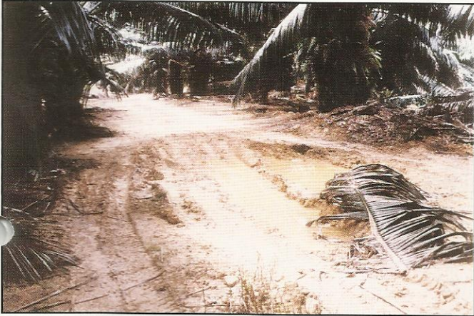
Plate 1. Initial condition of road surface
