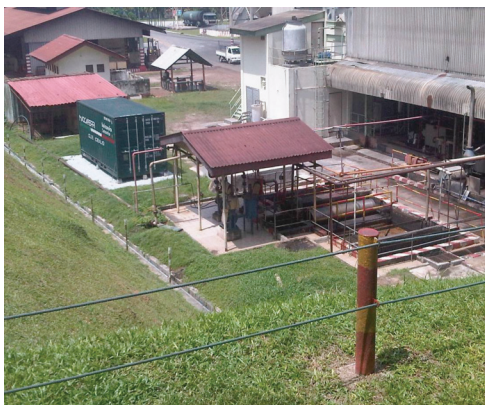
Figure 2. 'Oilsep' installed nearby the sludge pit.
