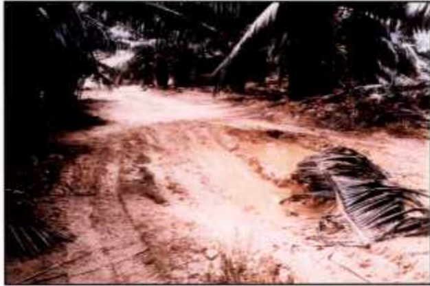
Plate 1. Initial condition of road surface
