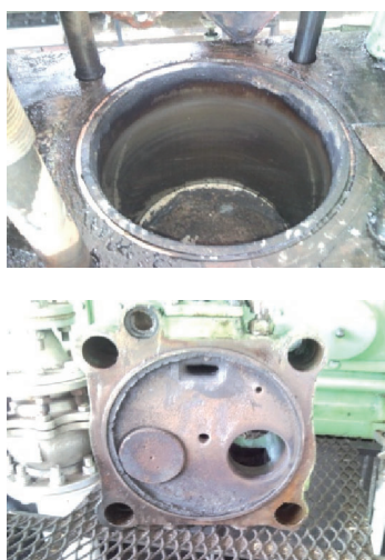
Figure 3. Condition of the combustion chamber of a gas generator using biogas for > 10 000 hr.
