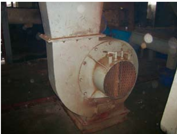
Figure 4. Adjustable damper controller.
