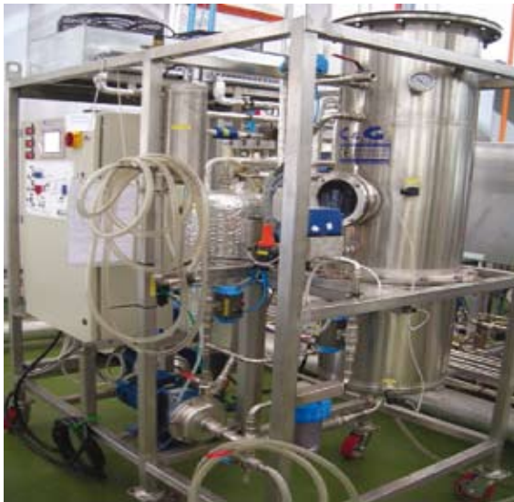
Figure 2. Pilot plant vacuum evaporator.
