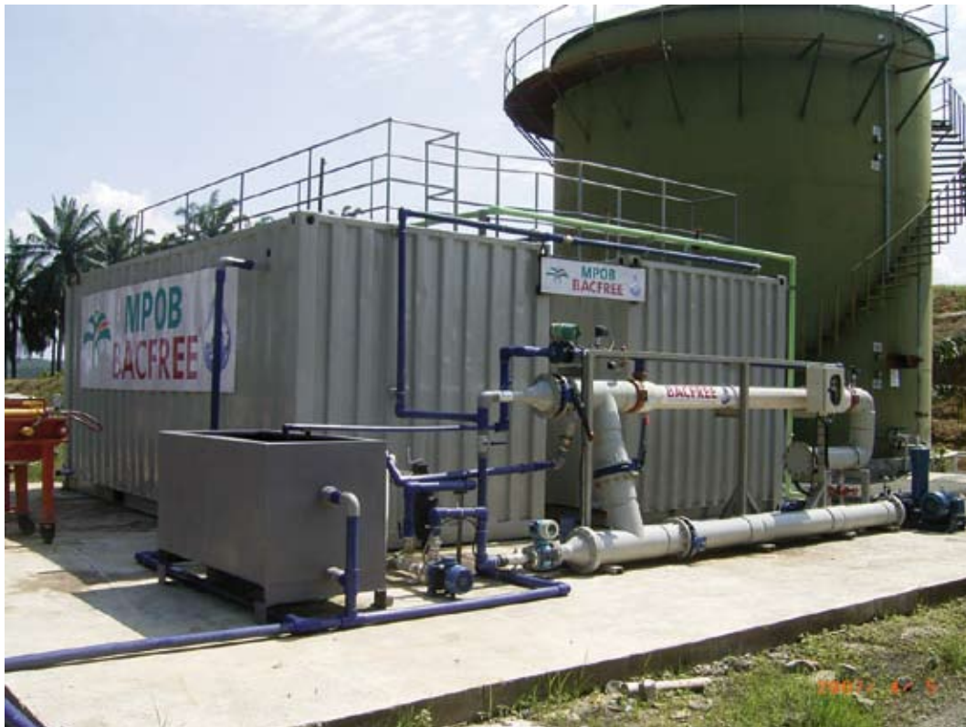
Figure 2. MBR pilot plant in POMTEC.
