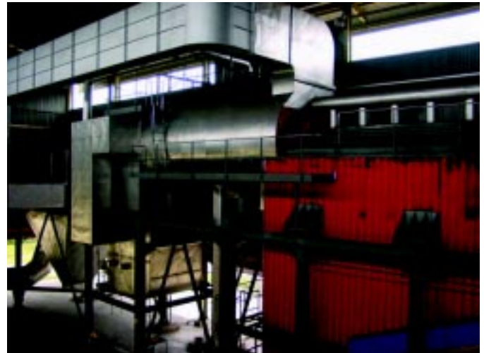
Figure 4. Fully automated boiler.
