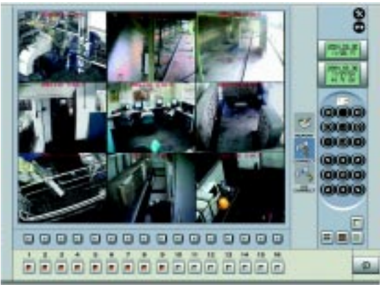
Figure 12. Closed circuit television (CCTV) system.
