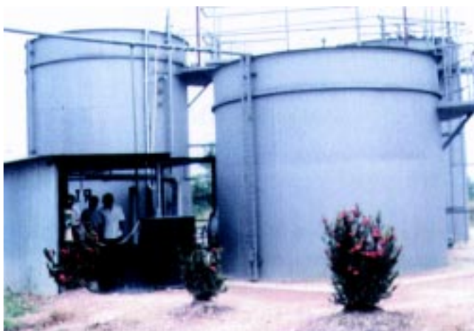
Figure 2. Commercial SBR Effluent Treatment Plant.
