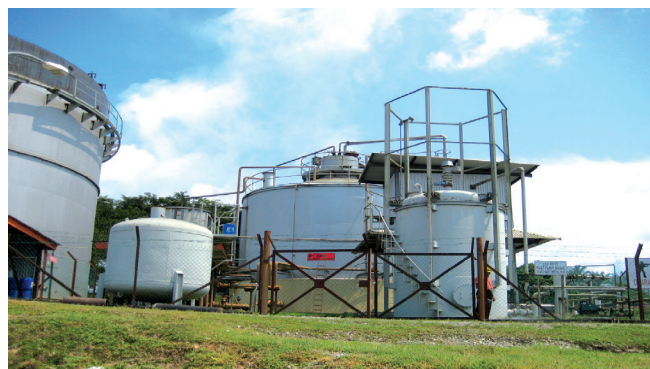
Figure 2. A POME digester tank to trap biogas at a palm oil mill.
