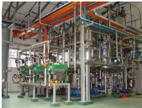
Figure 4. Refining pilot plant.
